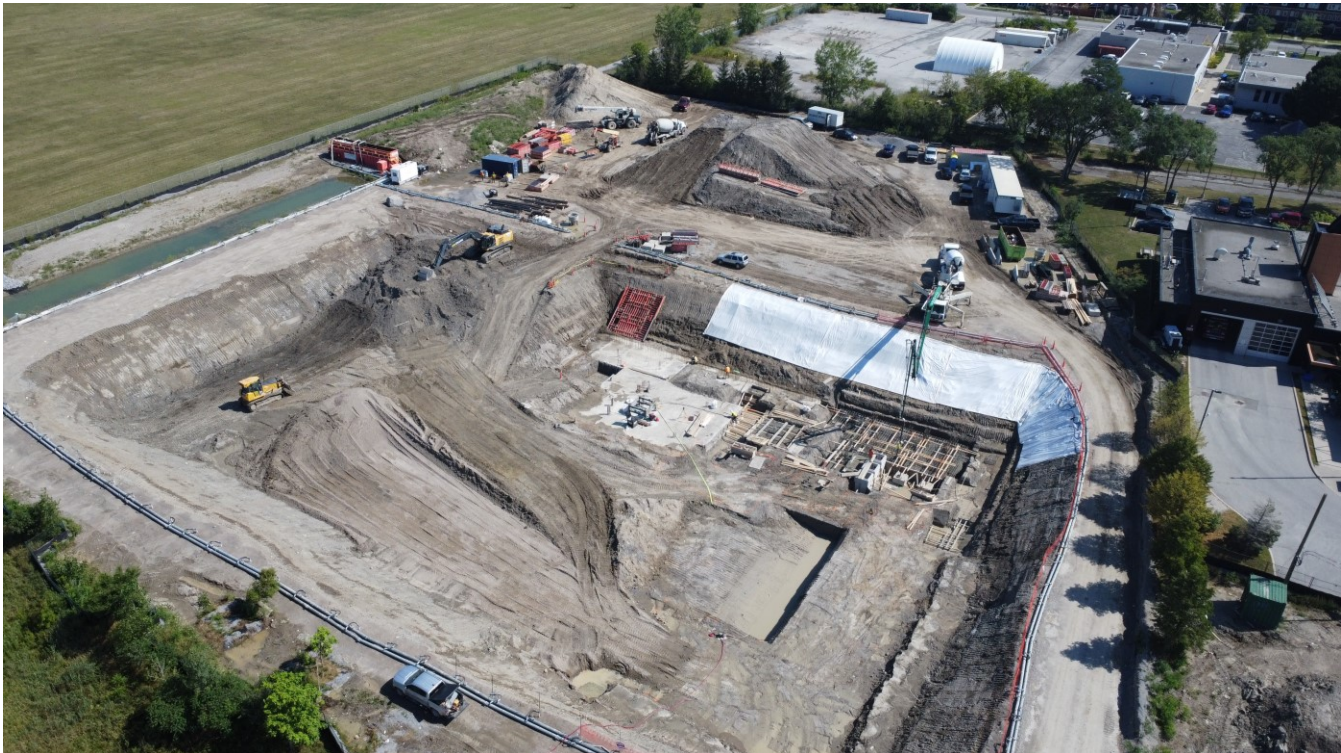
Above: the system functions very well to capture the groundwater across the interface. The excavation is completely dry and did not require any localized systems (i.e.: interior wellpoints) for the crane pad.
