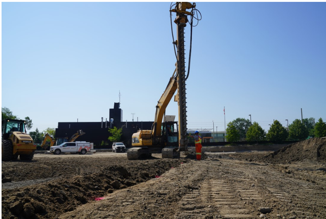
Drilling and jetting is performed in a small trench located outside of the proposed building footprint to control the water and spoils. Tracked mud is not permitted from site access roads to City of Toronto roadways.
