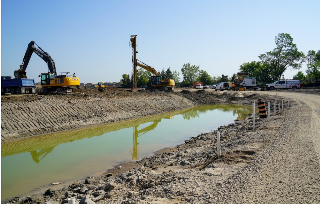
A temporary trench was excavated at the north end of the site to confirm the groundwater level.
